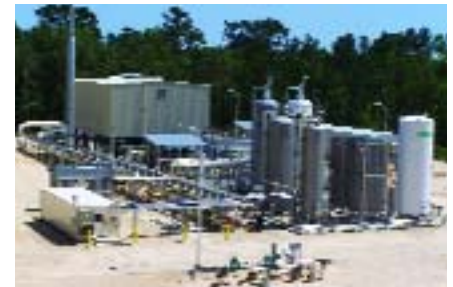
Integrated cavern support equipment.
